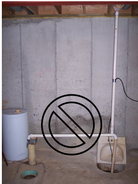
FOOTING DRAIN PUMPED INTO SANITARY SEWER
