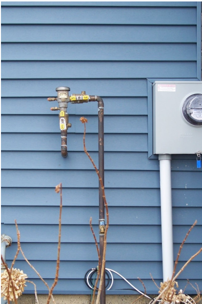
LAWN SPRINKLING PRESSURE VACUUM BREAKER
